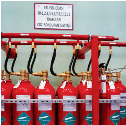
Sample of High Pressure CO 2 System
