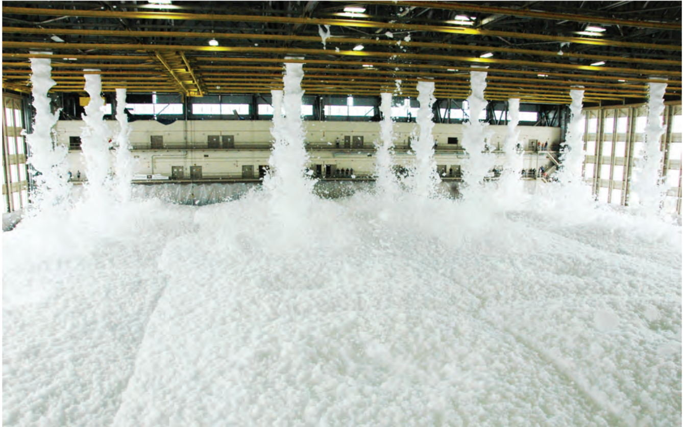
Aircraft Hangars High Expansion Foam Extinguishing System
